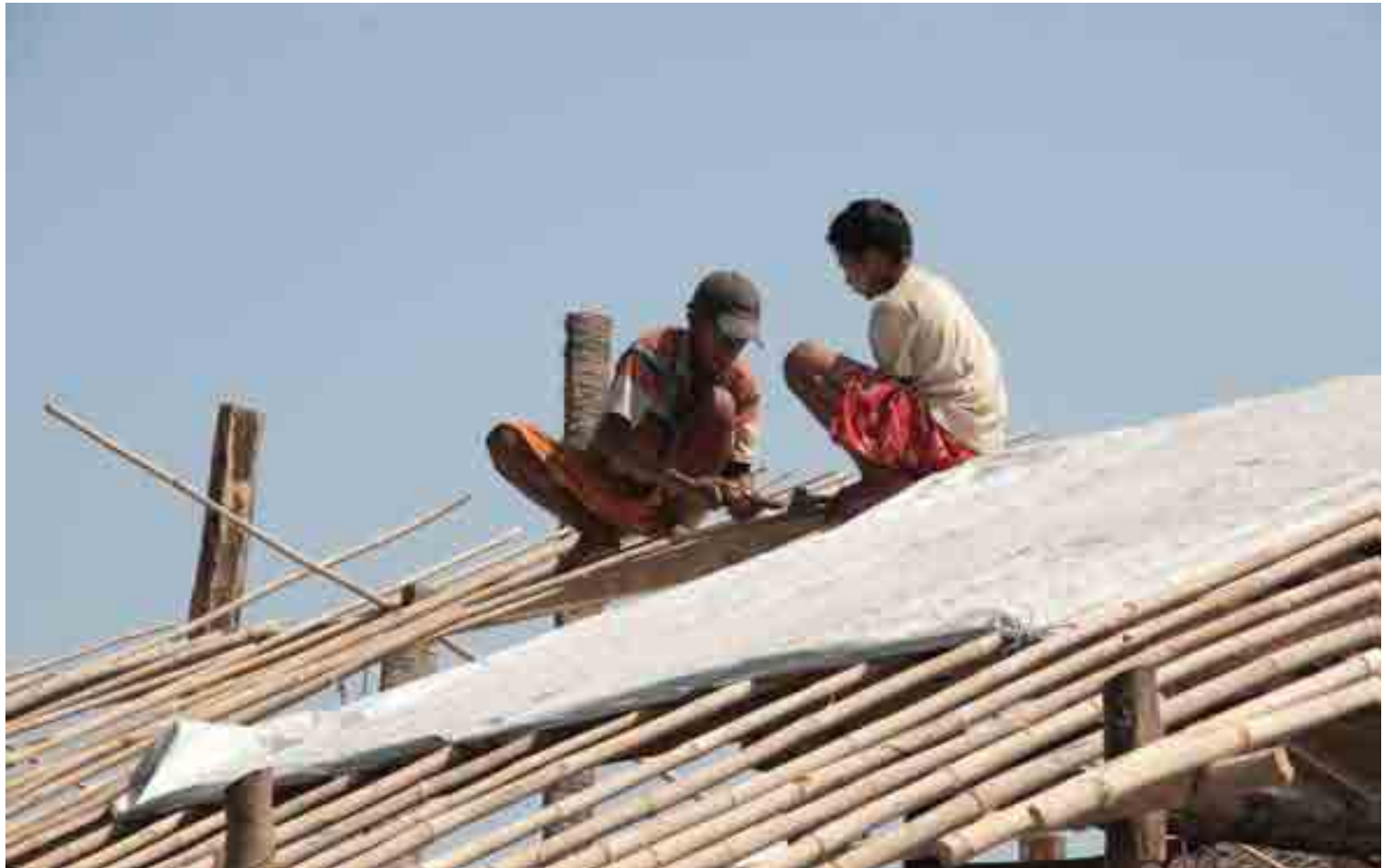
Villagers from Kinwon Village, Pyapon repair their households. Photos by AHTF Coordinating Office
